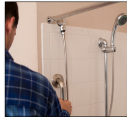
We install grab bars for safety.
