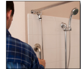
We install grab bars for safety.
